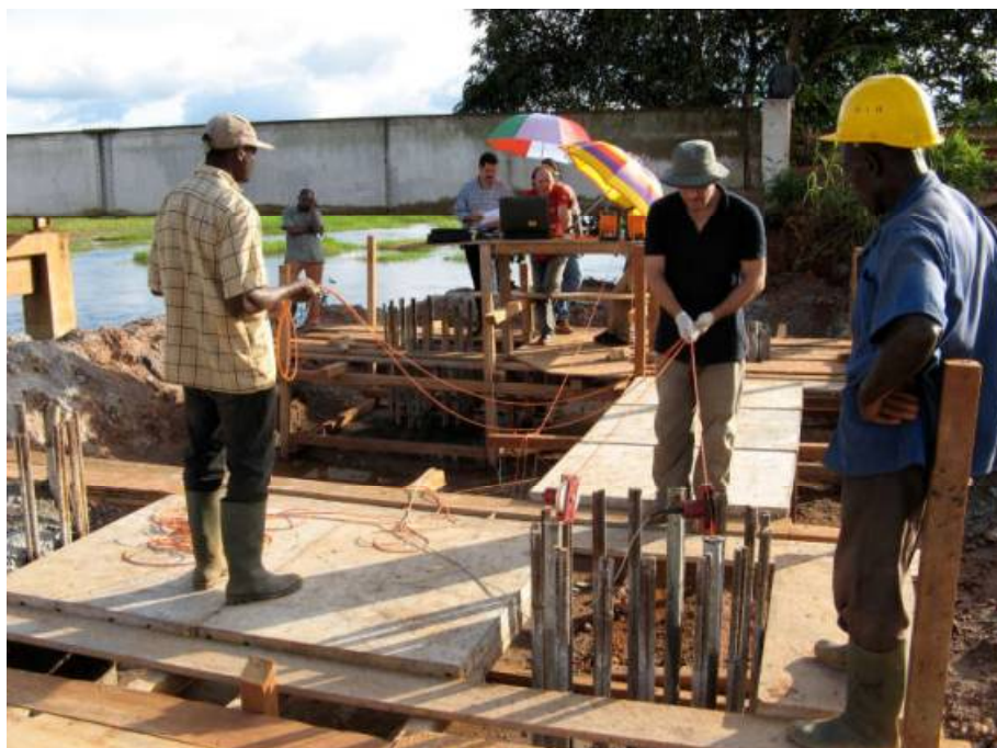
Performing Ultrasonic Tests on pile foundation of a bridge at the Melong - Dschang road in Cameroon
